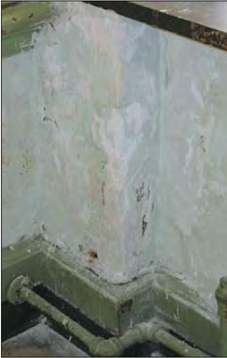
Age and neglect have left the walls in some schools—like this New York classroom—literally crumbling.
